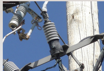
Distribution Cable Joints
