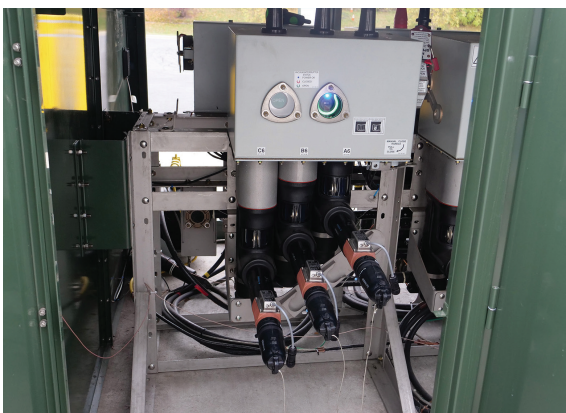
Underground platform with product installed (VS-27-UG)
