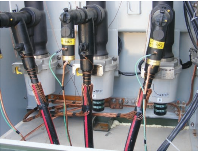
Viper-ST reclosers, adapted for dead-front, are in the 12-kV side of the transformer enclosure; elbow arresters are connected to the T-Ops.
