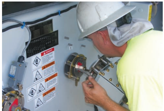
The 35-kV switchgear has a remote switch mechanism to allow the operator to switch from up to 50 ft away from the gear. Lineman Merrill Colby attaches the mechanism to the gear.
