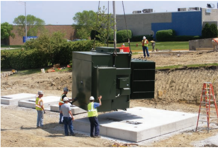
The 34.5-kV to 12.47-kV dead-front transformer is lowered onto the precast pad as crew members prepare for proper placement.
