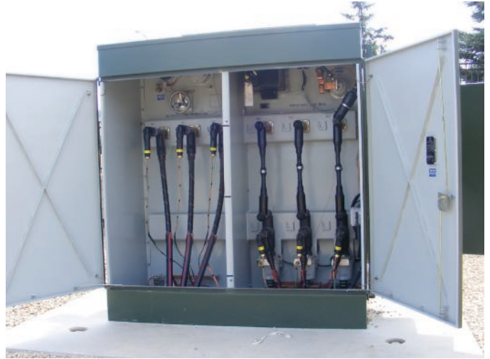
All cable connections are dead-front inside the 34.5-kV (left) to 12.47-kV (right) pad-mounted transformer.
