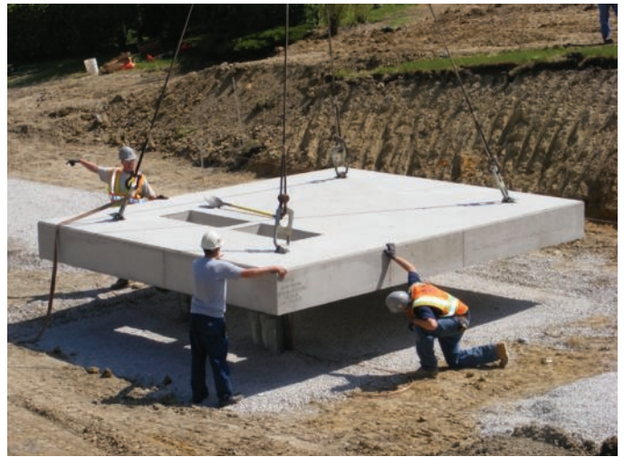
The crew set the 50,000-lb transformer pad just minutes before the transformer.
