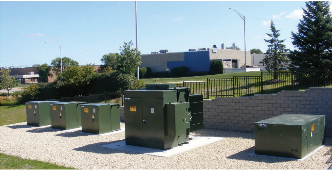
St. Charles' LDC #1 sits on landscaped area provided by the industrial customer. The components (left to right) include three pad-mounted voltage regulators, a 34.5-kV to 12.47-kV dead-front transformer and the 34.5-kV switchgear.
