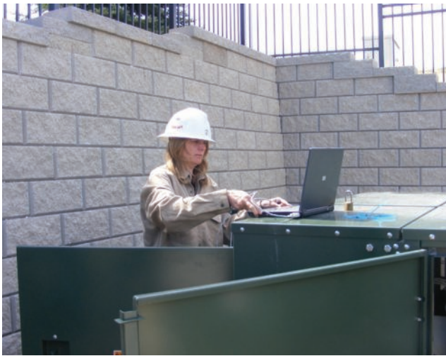
St. Charles substation engineer Erika Drennen uses a laptop to program the relays in the control enclosure attached to the 35-kV gear.
