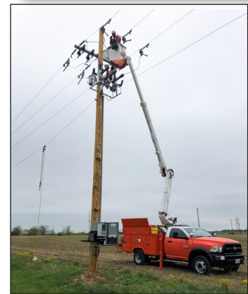
Viper-ST recloser with 6 Voltage Sensing, control power transformer, 900 MHz radio and SEL-651R control.
