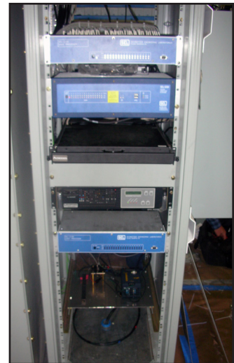
The SEL 2100 processor is rack mounted in a nearby equipment room.
