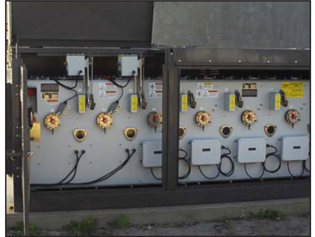
Six way padmount switch with motor actuators on source ways 1 and 2.
