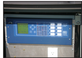
The SEL 451 relay is housed in a separate enclosure on the side of the switch.
