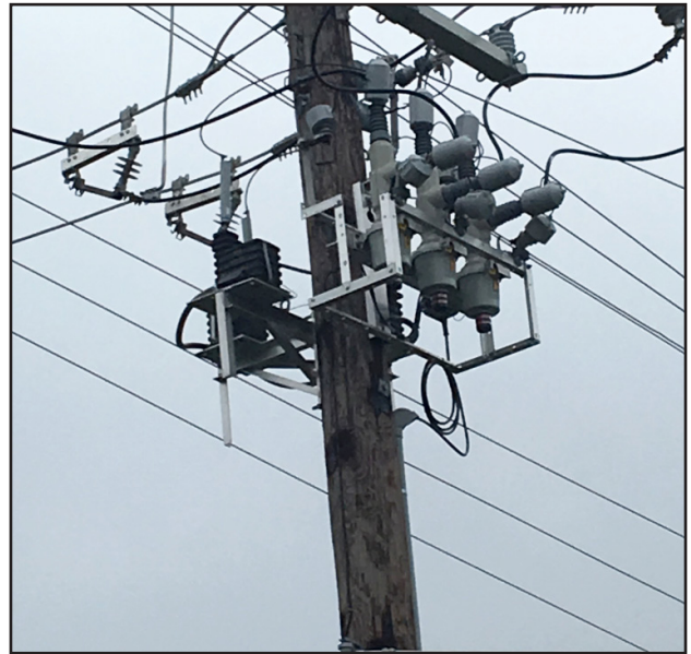
Before: Existing Viper-ST Installation
