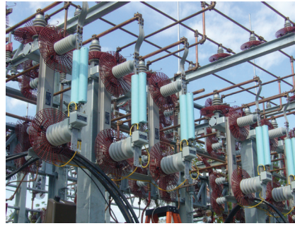
University substation outdoor installation
