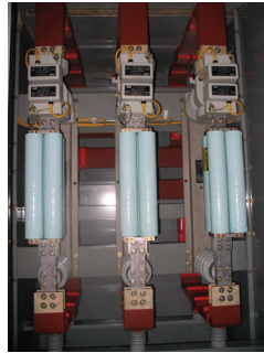
Three-phase system in an enclosure protecting an FPSO
