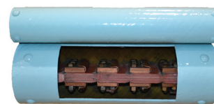
Close up of the severed main conductor and melted current limiting element of a 3000A (double bus) CLiP after interruption
