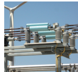
CLiP protecting the substation of a midwestern windfarm
