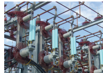
CLiP installed in a generating station at a large southeastern university
