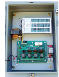
Control box with inverter
